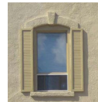
Narrow shutters are not in scale with window width appear inoperable.
